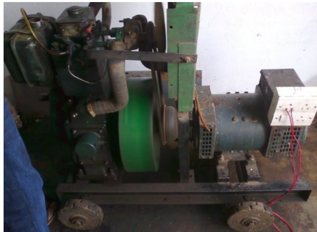
Fig 1: Diesel generator set used for the test
